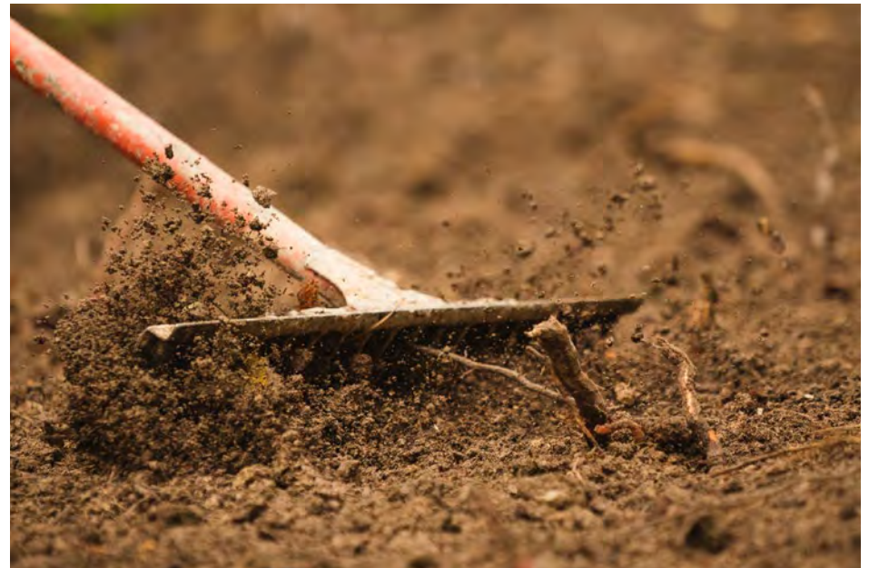
Trail construction employs a host of advanced tools, but sometimes the job simply calls for the time-tested rake.
