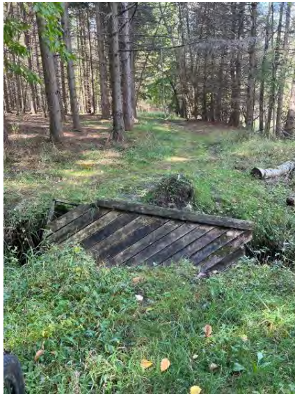
Bridge in disrepair; trail should be decommissioned.
